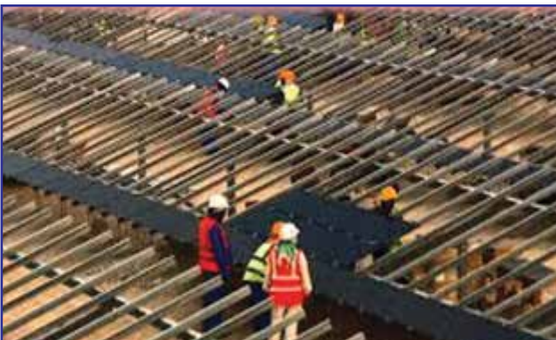
HH SHEIKH MOHAMMED BIN RASHID AL MAKTOUM SOLAR PARK
