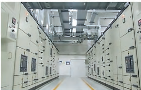
Main Distribution Board
