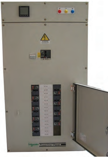
Sub Main Distribution Boards
