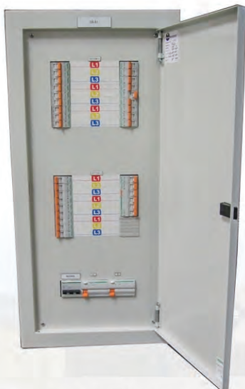
Final Distribution Boards
