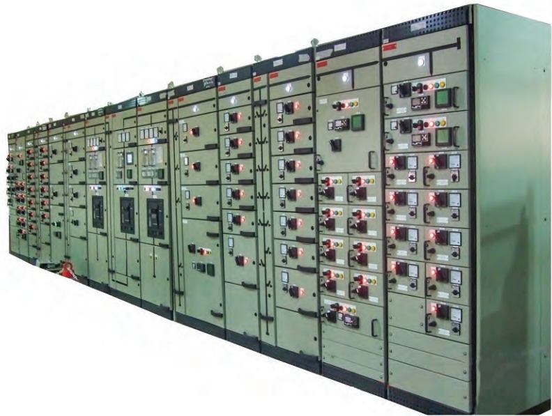
Motor Control Centers
