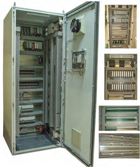
Programmable Logic Controller (PLC)
